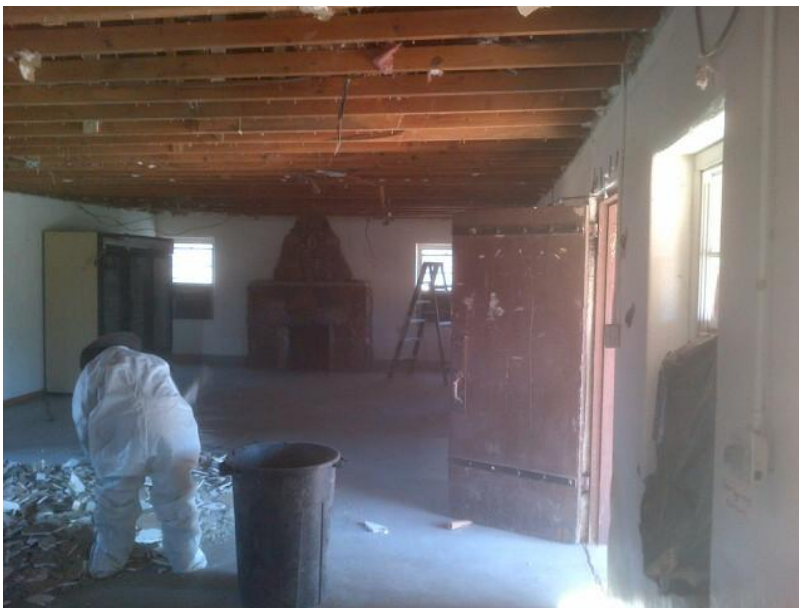
The building nearly gutted
