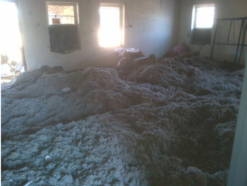
Insulation cleaned out of the ceiling covers the floor
